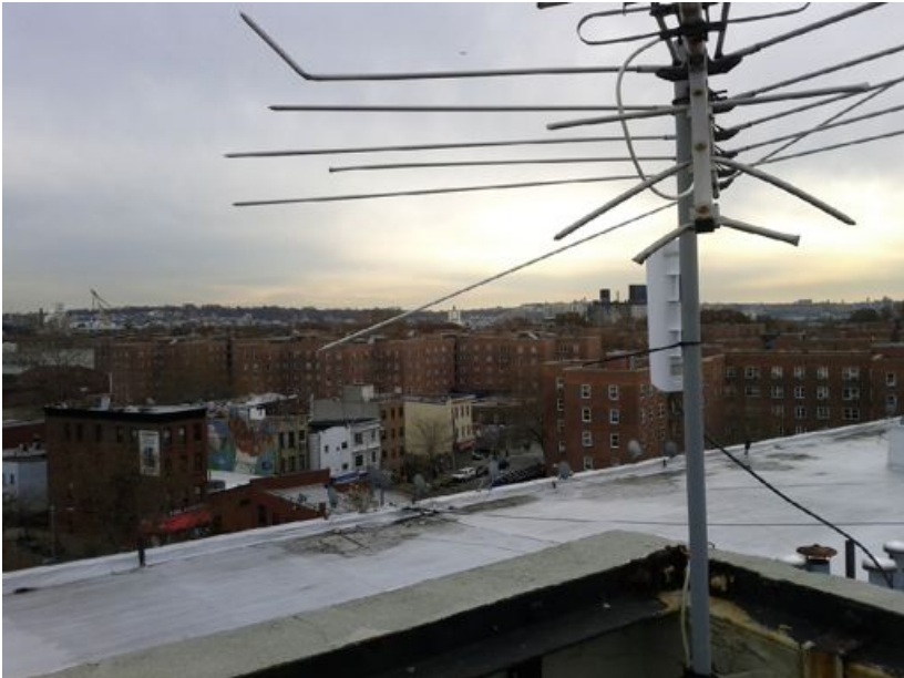
Figure CsOTI 13: Rooftop node. In the aftermath of Superstorm Sandy, additional community members offered to host RHI WiFi nodes and a local ISP donated Internet connectivity.
