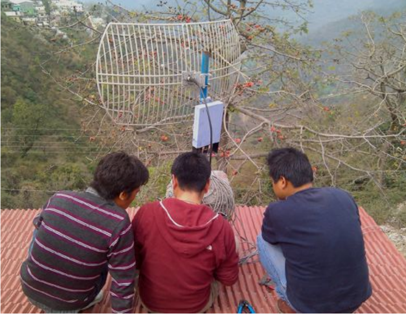
Figure CSD 6: Relay troubleshooting, Kumaon Network
