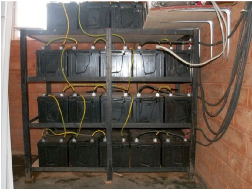
Figure OGP 9: A battery bank of 3600 Ah, currents reach levels of 45 A during charging
