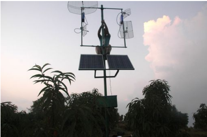
Figure CSD 7: Last touches to solar relay, Kumaon Network
