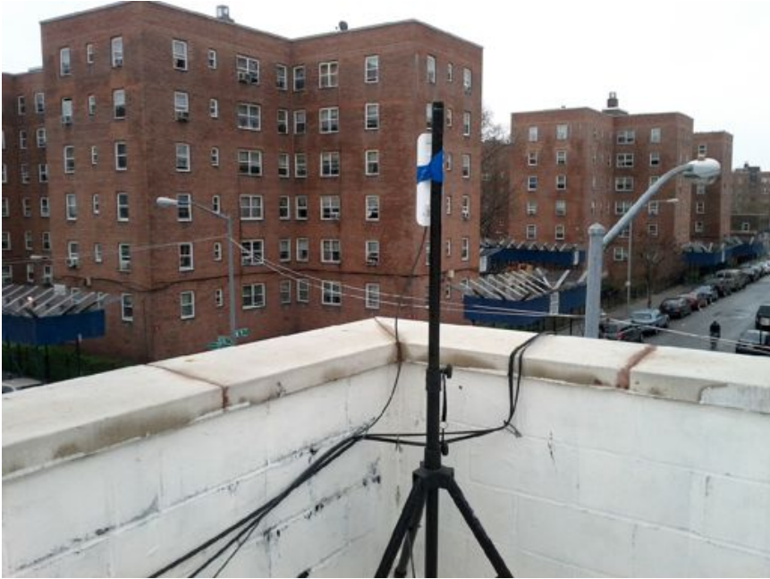
Figure CsOTI 4: First RHI WiFi node (Ubiquiti Nanostation) installed on the rooftop of the building that houses the RHI offices.
