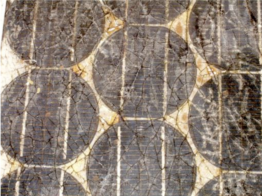
Figure OGP 6: The effect of water and corrosion in a solar panel
