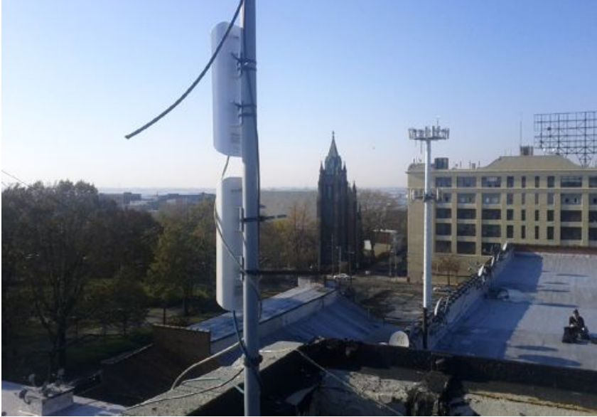
Figure CsOTI 14: Rooftop node installed after Superstorm Sandy.
